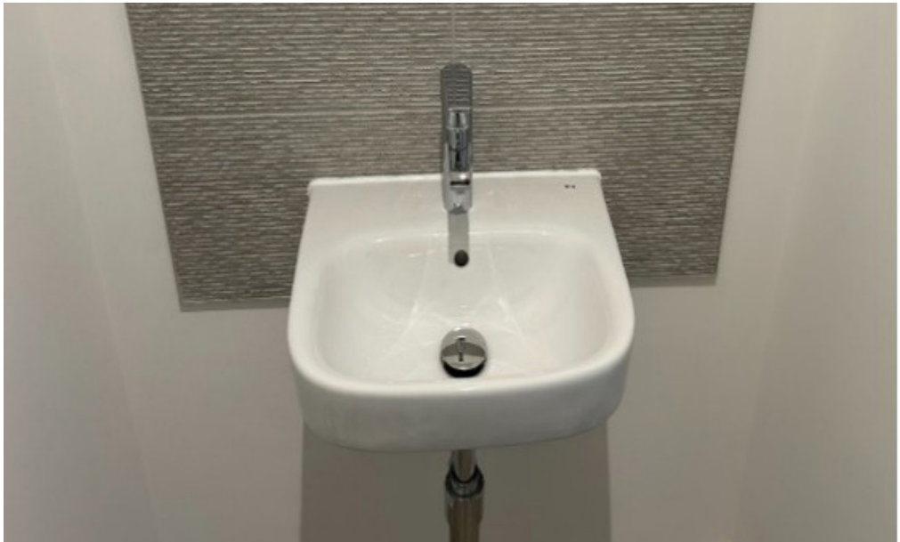
Examples of neat and well-presented sanitary fixture installations.
