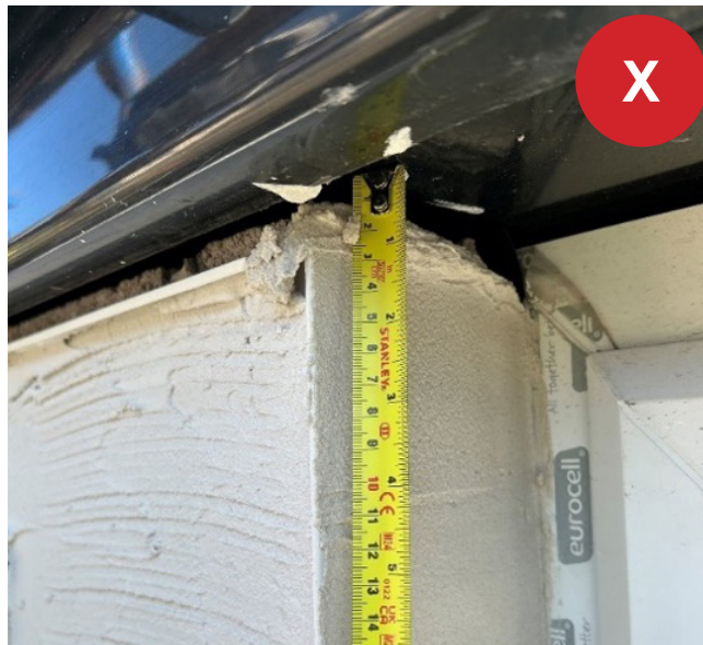
The gap left between the top of the external masonry and the underside of the soffit is not enough to facilitate the expected settlement at this location.
