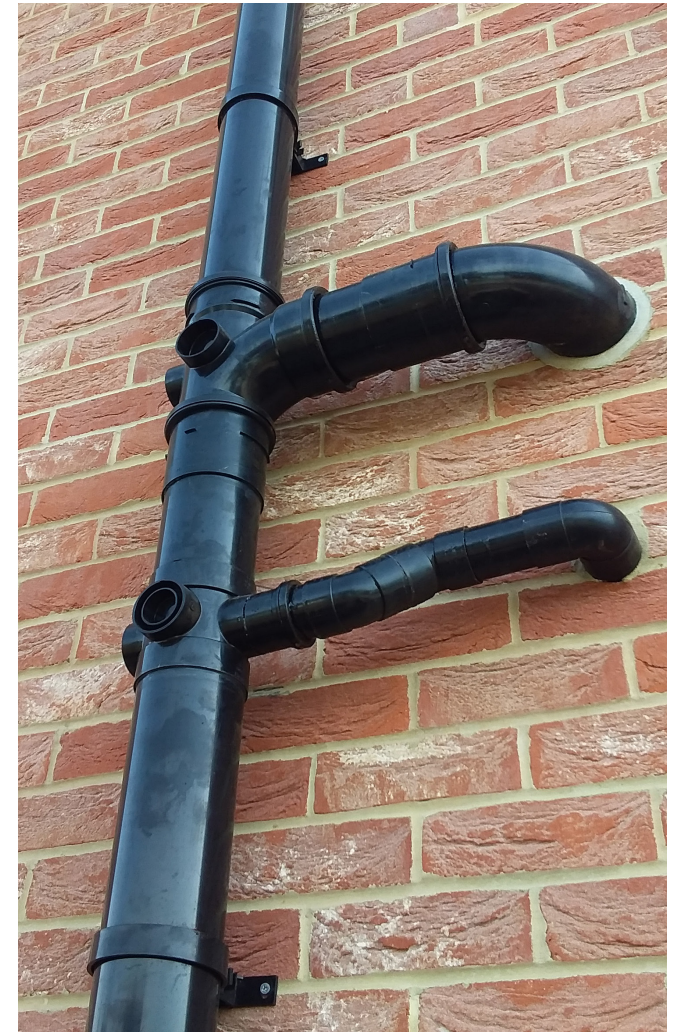
A neatly arranged series of branch connections into the SVP stack. Penetrations through the masonry have been neatly formed and well sealed.
