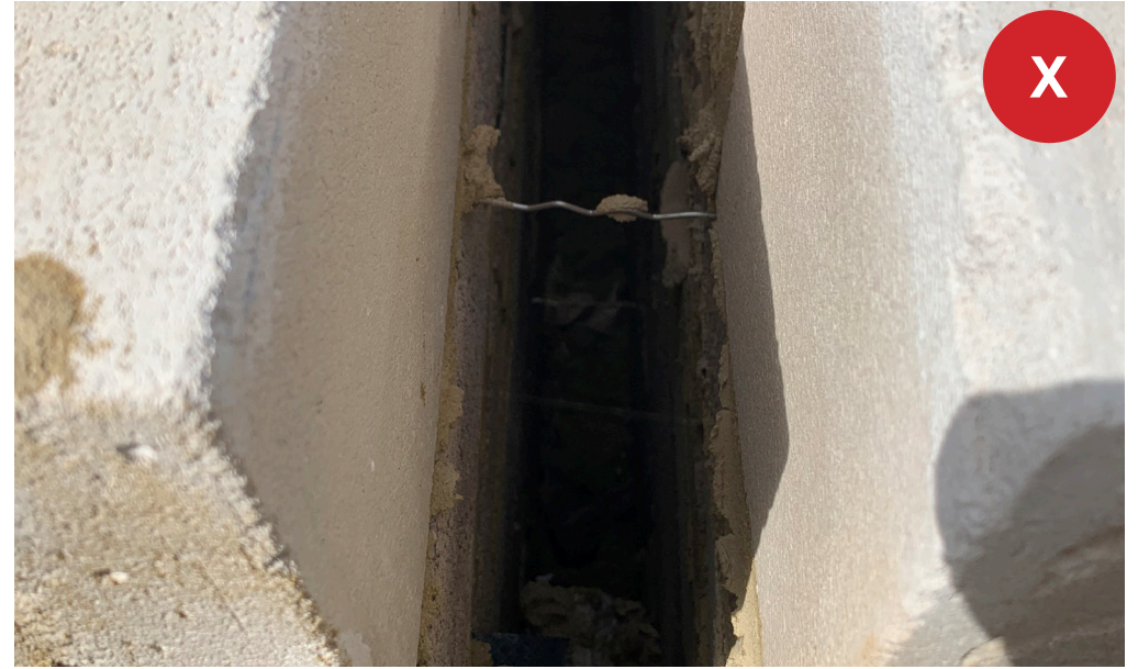
Mortar debris has been allowed to drop into the cavity sitting on wall ties and DPC material protruding into the cavity.
