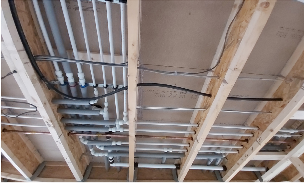
A neat pipe work installation with pipe support set at regular intervals utilising proprietary metal brackets. Sanitary pipe work passing through joist positions has been sleeved with felt fabric to allow thermal expansion to occur unhindered and without the risk of associated noise.
