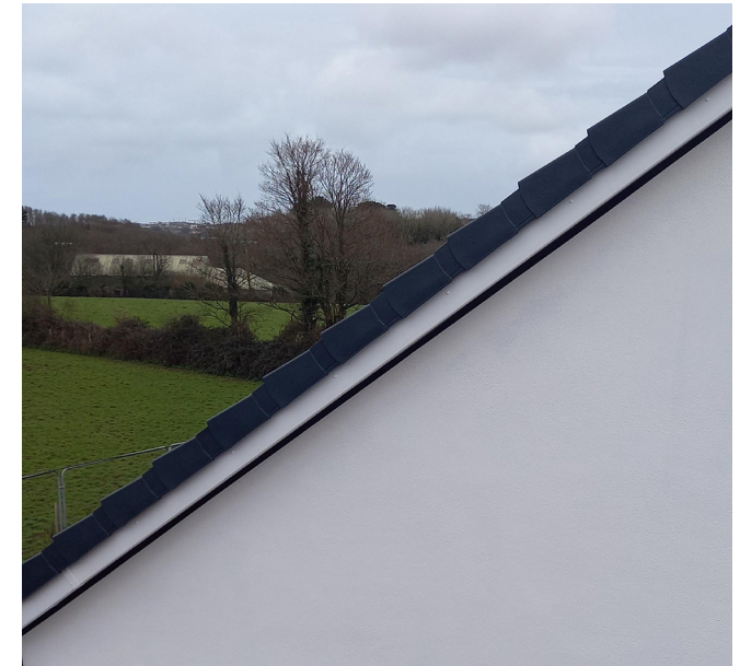
This rendered gable has a differential settlement gap between the completed render stop bead and the soffit at the roofs verge. When settlement occurs, the gap will close up. The attention to detail on display here is that the exposed masonry in the gap has been painted black rather than left as a bare concrete surface.
