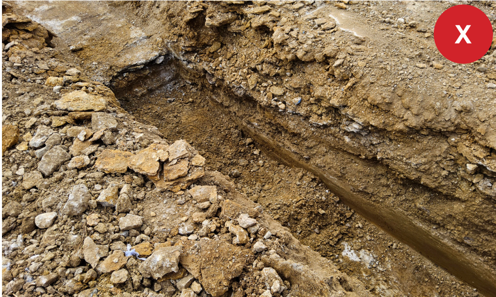
A stepping excavation being affected by the strata. Loose material and a loss of strata in the sides of the excavation and collapsing of the step detail. This required further attention to bring up to the required standard.
