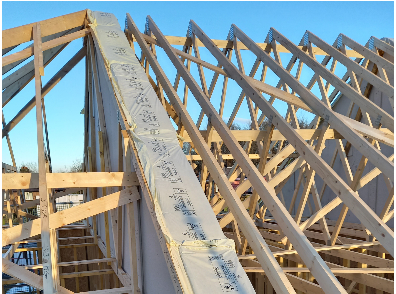
A proprietary polyethylene sleeved fire stopping product installed over a compartment wall spandrel panel. The spandrel panel has been set to ensure the fire stopping finishes touch tight with the roofing underlay material.
