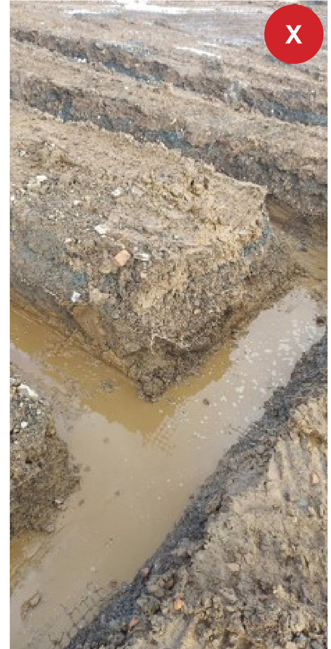
Overnight rain has resulted in standing water within an excavation. This needs to be cleared and the excavation scraped and cleared of any debris and spoiled strata before any concreting takes place.
