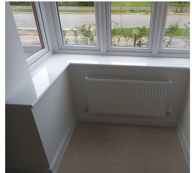
Painted surfaces free from noticeable runs, dust, and brush marks.
