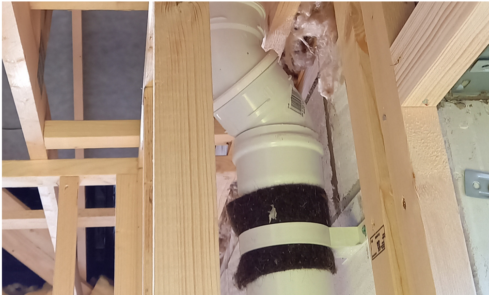
An SVP secured and supported by a proprietary bracket. A felt fabric has been placed to ensure any thermal movement in the pipe is not restricted.
