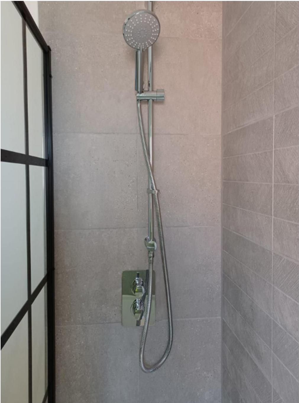
Examples of neat and well-presented installations.
