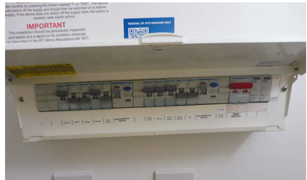
A labelled consumer unit fitted with blanks. MCBs and RCDs are accessible and operational, and the cover fully secured.
