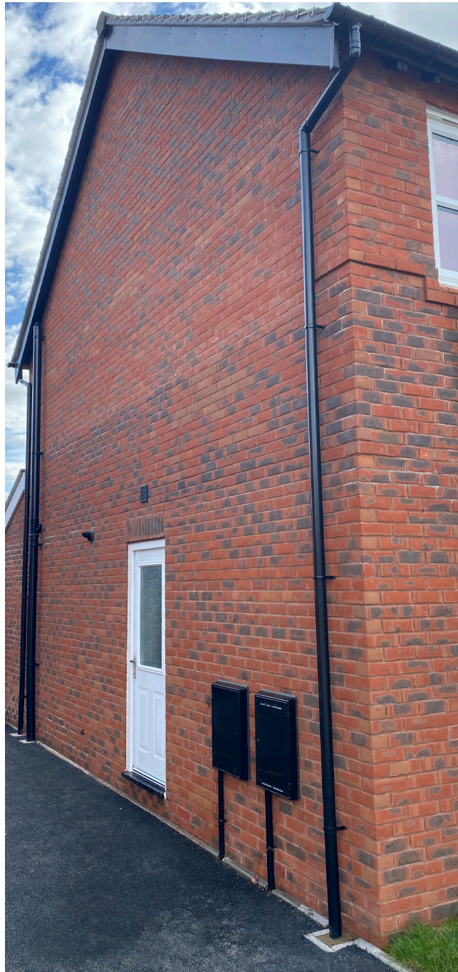
A rainwater down pipe secured at 1.8m centres using proprietary clips.
