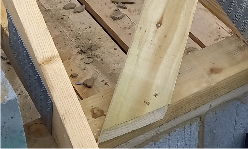
A diagonal bracing has been correctly nailed at its union with the wall plate.
