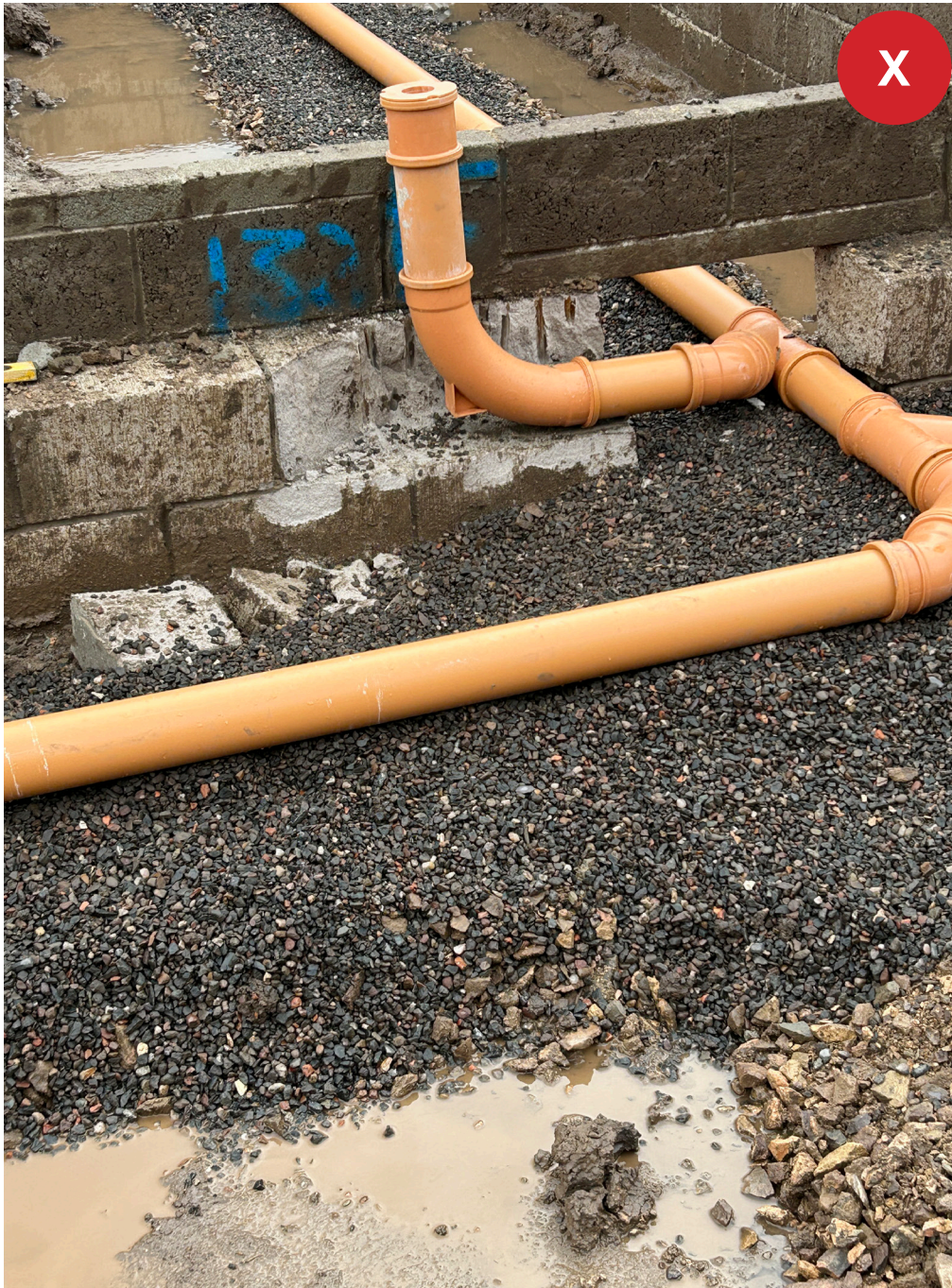
The substructure masonry conflict with drainage was incorrectly resolved by breaking out material, requiring additional work to restore the masonry to the required performance level.
