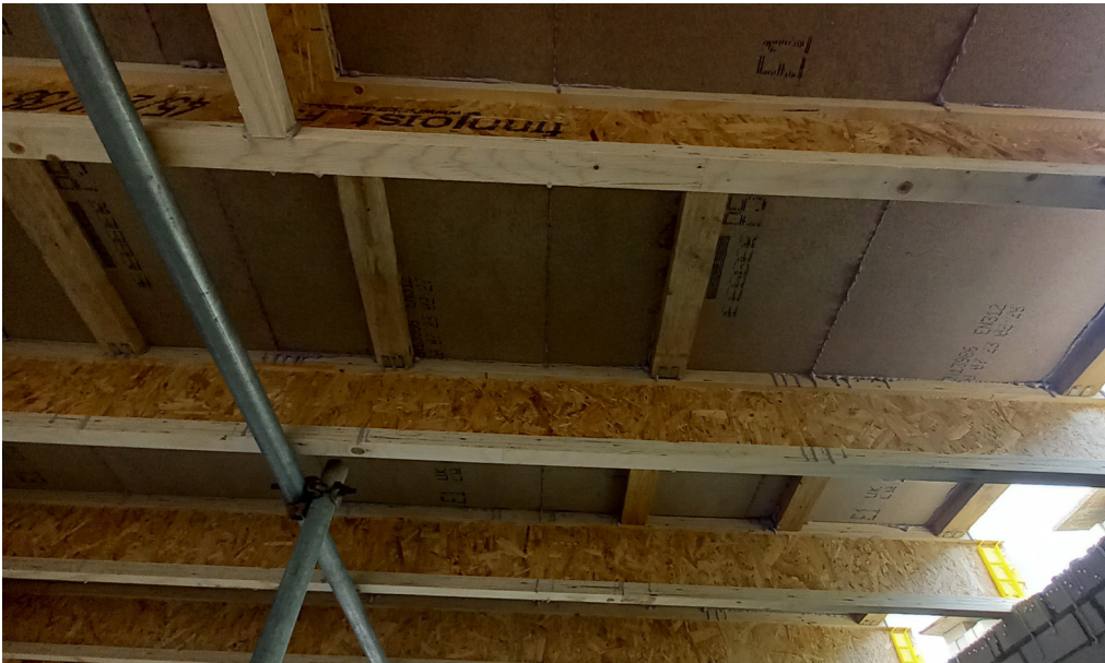
Bridging noggings have been correctly provided at right angles to joist span direction to support a non-load partition located above.
