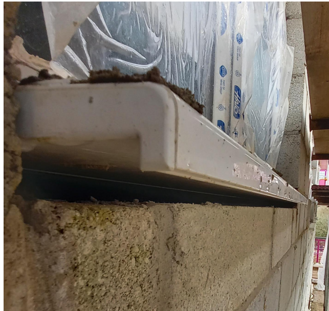
Allowance for movement between the timber frame and the external masonry has been provided underneath this sill location. The materials used to fill the final gap should allow for settlement in the timber frame due to shrinkage.
