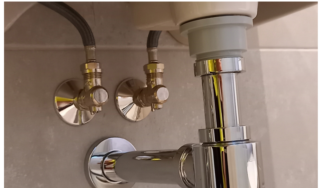
Neat waste fittings. All pipework appropriately concealed e.g. neatly fixed behind the sink.
