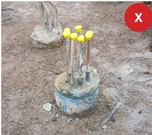
Trimming down to the pile heads has been commenced with one pile head suffering significant damage during the work. The condition of the reinforcement would need to be assessed by an engineer and a remedial plan proposed and agreed to rectify the situation.
