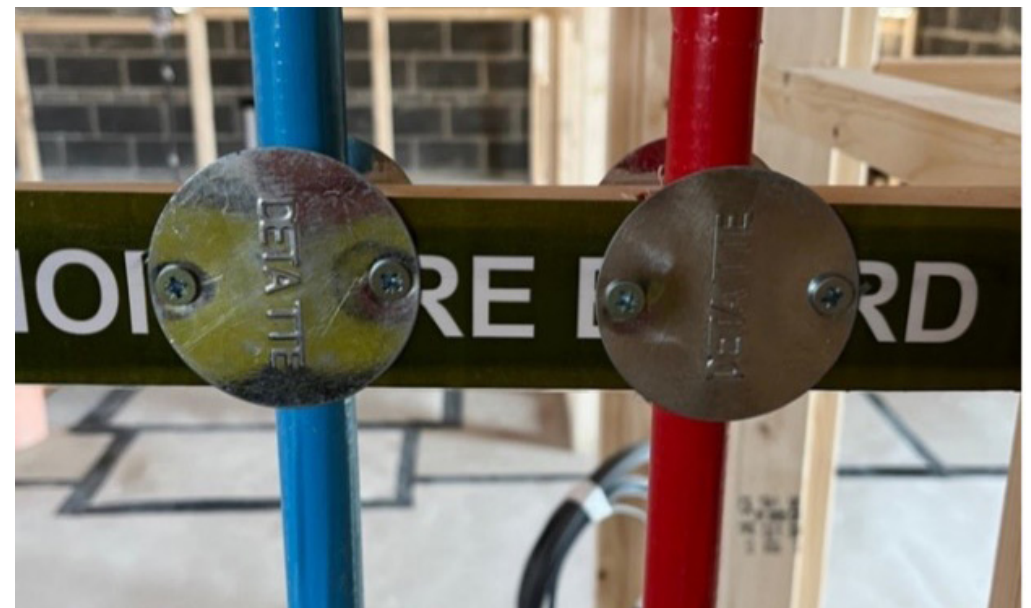
Pipes being protected by a metal plate to safeguard against potential fixing strikes.
