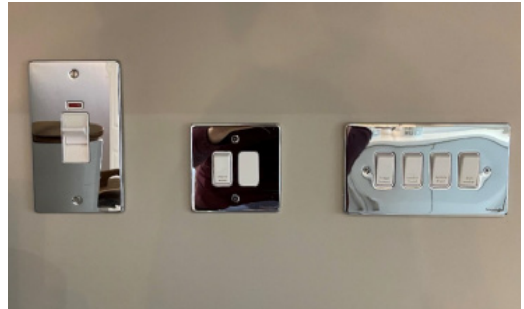
A series of switches – neatly aligned and spaced, and square and level.
