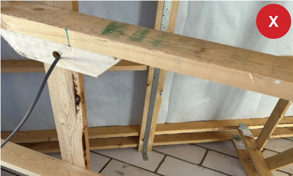
This arrangement has the lateral restraint incorrectly surface fixed into masonry instead of being located through a perpendicular mortar joint and 'hooked' within the cavity at a full block.
