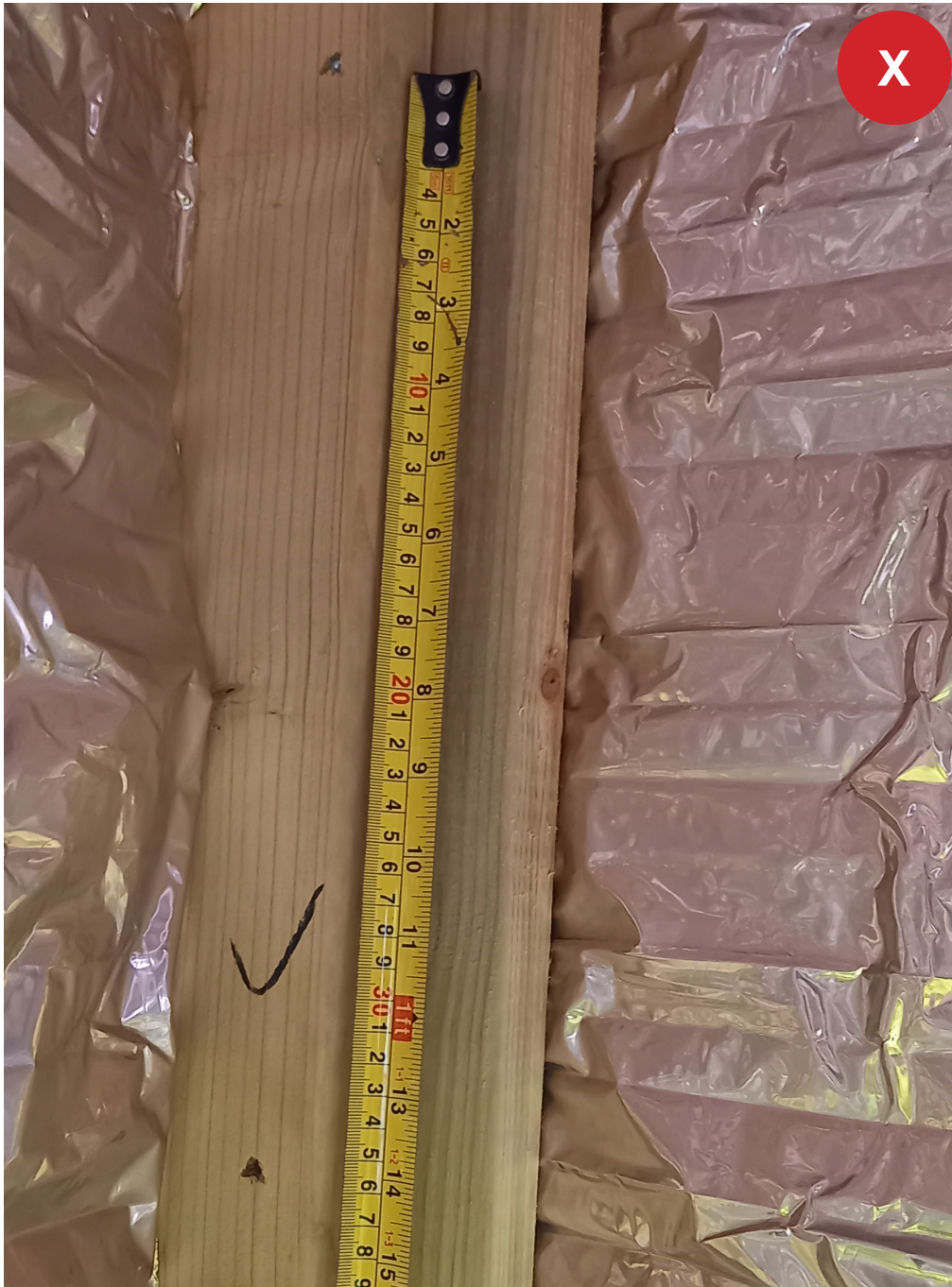
Fixings at corner junctions between panels were noted to have drifted beyond the 300mm specified by the engineer. Additional fixings would be required on a revisit to rectify.
