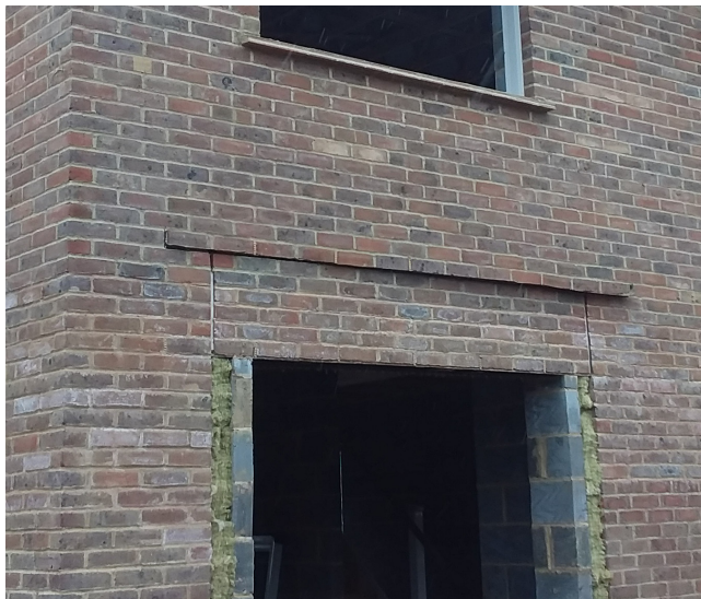
On this bay window construction, the cavity tray has been left to extend out through the external leaf of masonry to ensure the abutting flat roof construction water upstands finish under its location. A vertical DPC has been installed at either end to ensure moisture cannot flank around the roof construction where it abuts the masonry.
