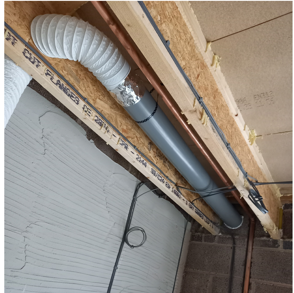
Well supported rigid duct work with a short section of flexible pipe used for final connection. The penetration through the external wall is neatly formed and sealed.
