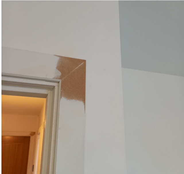
Architraves neatly fitted. Even margins with joint surfaces smooth, clean, and free from damage and excessive filler.
