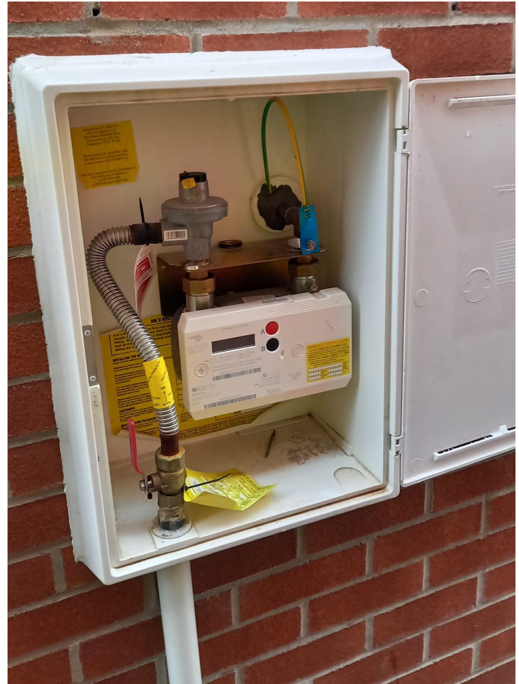
Sealant used around the meter box perimeter is well executed, and smooth and free from gaps and smears. All penetrations are sealed. All safety features such as shut off valves and earth bonding clearly visible.
