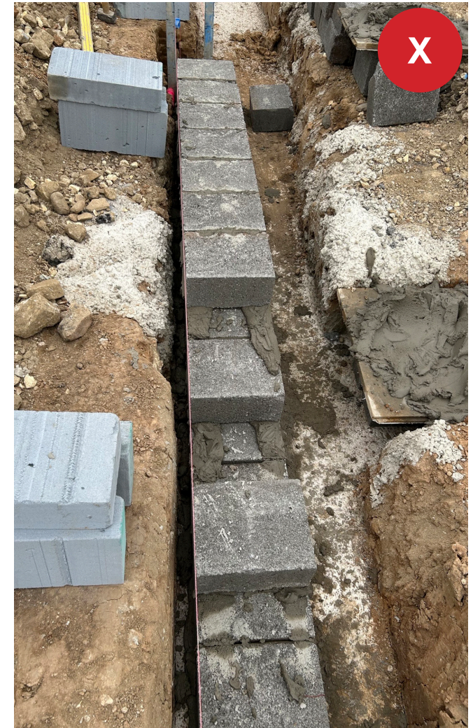
Setting out work has been carried out incorrectly. The centre line of the substructure masonry should be aligned with the centre line of the foundation
