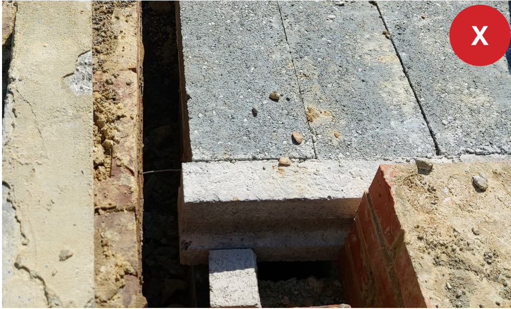
Beam ends have been allowed to encroach into the cavity. When coursing units are laid, these ends are at risk of creating ledges within the cavity for mortar debris.
