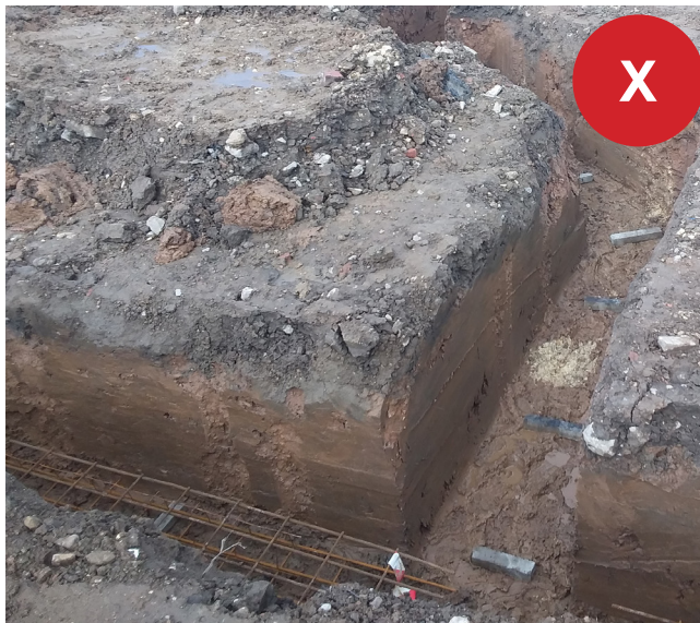
The excavation base has been churned up by foot traffic. Concrete spacers have been pushed into the supporting strata losing any chance of providing the required cover and support.
