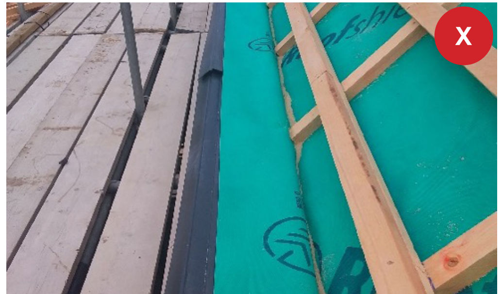
An incorrectly formed eaves detail on this counter battened roof has resulted in a water 'trough' being inadvertently created behind the fascia board.
