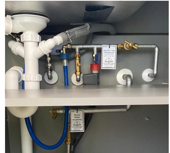
All pipework is neat and well presented. Accessible shut off and isolation valves have been tagged and located to ensure easy access and operation when required.
