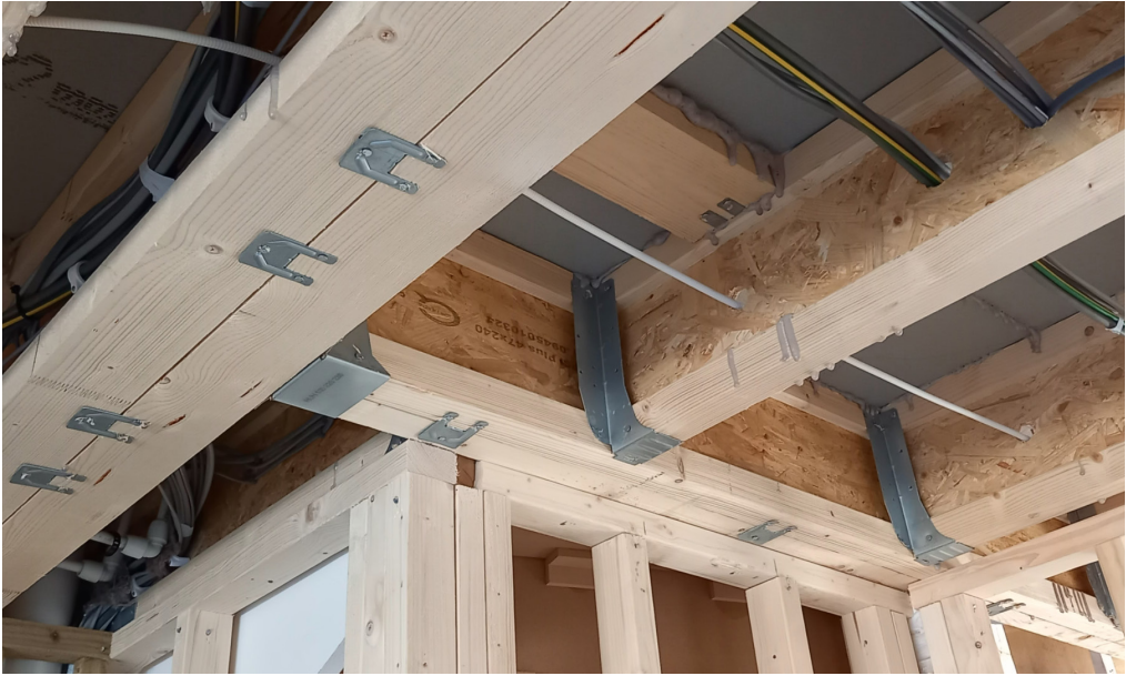
Load sharing metal connectors are installed on these I-joists to promote even load distribution across these adjacent joists. This improves stiffness, stability, and mitigates the effects of potential movement between joists.
