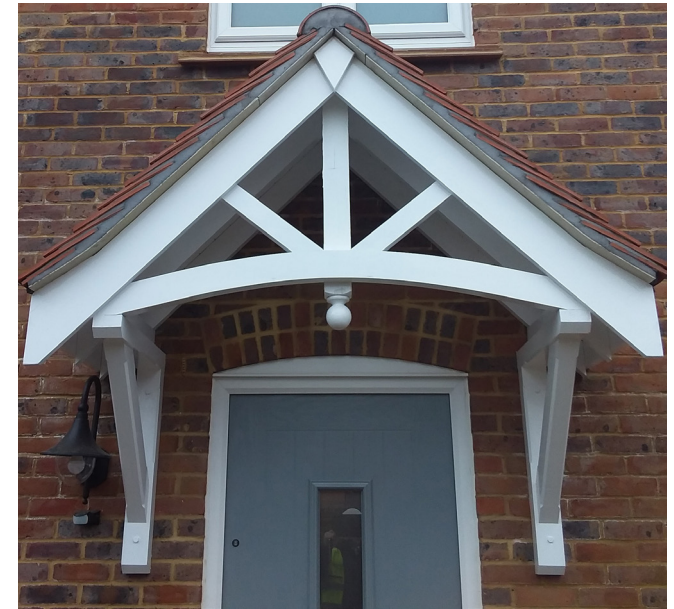
A large, tiled canopy – it is essential that such elements are securely fixed to a site-specific design specification. The specification should detail the type, size and material for brackets. Fixings must be suitable for the substrate type and capable of withstanding foreseeable loads e.g. dead load, wind, and snow.
