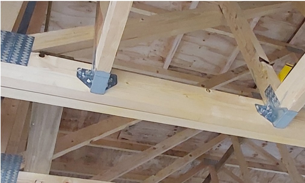
Proprietary truss hangers fixed onto a multiple trussed rafter arrangement. Hangers are fully nail fixed.
