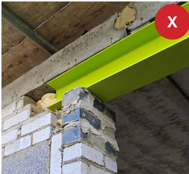
Very poorly constructed supporting masonry to a large structural steel beam. This position should have included a padstone and the masonry around it built bonded and fully secured.
